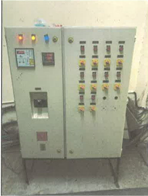
Various electrical Parameter of the system
