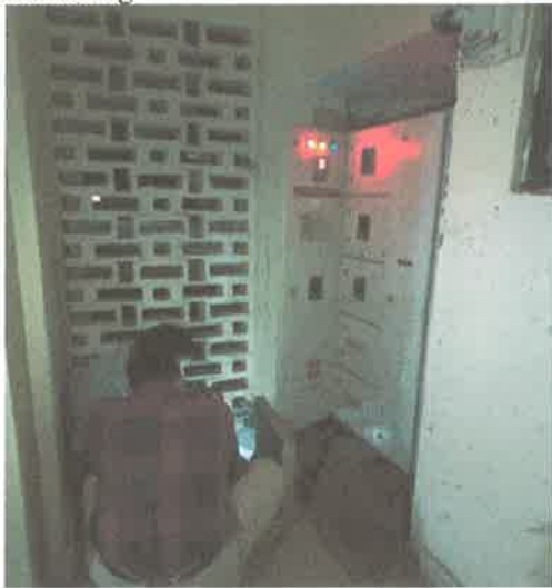
Various electrical Parameter of the system
