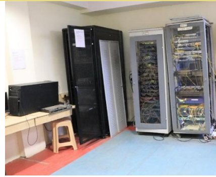
Fibre Terminating Rack and Server Room
